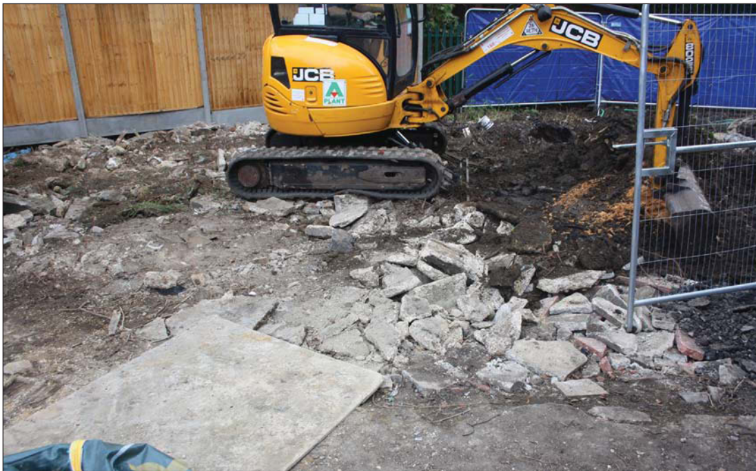
Plate 2. Wet ground at south of site, looking south.
