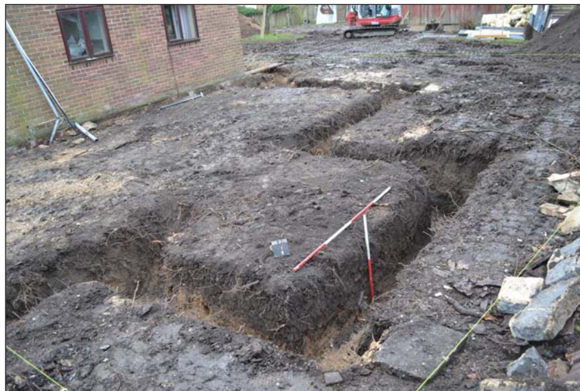
Plate 1. View of new footings to north of existing house, looking south east, Scales: 2m and 1m.
