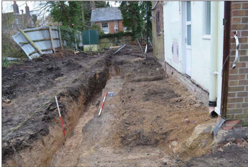
Plate 3. View of new footings to east of existing house, looking south east, Scales: horizontal 2m, vertical 1m.
