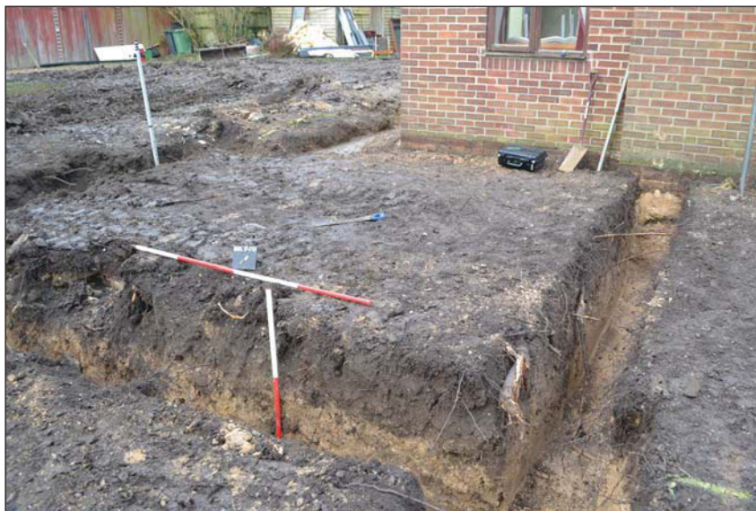
Plate 4. View of new footings to south of existing house, looking north north west, Scales: horizontal 2m, vertical 1m.
