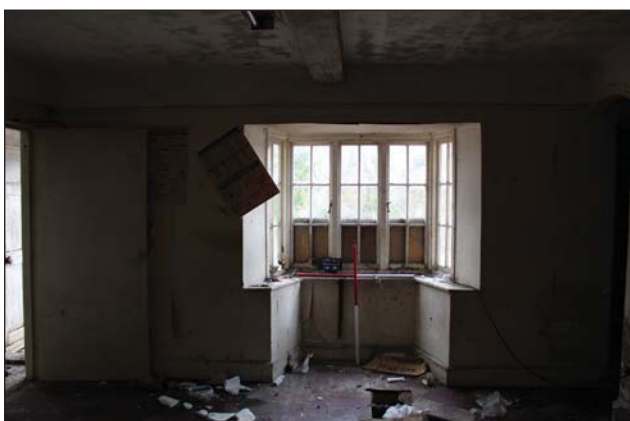
Plate 13. Old School House, Room 2, View to bay window, looking NW, Scales: 2 x 1m.
