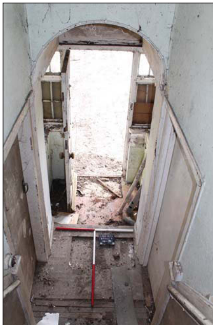
Plate 7. Old School House, hall, View to porch, looking NW, Scales: 2 x 1m.
