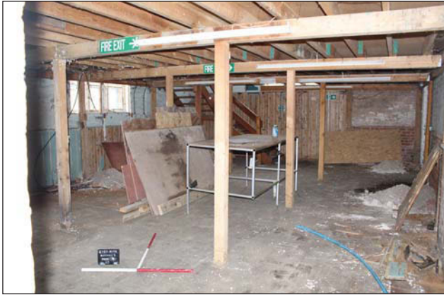
Plate 31. Former School, Room 2, General view to stairs, looking E, Scales: 2x 1m.
