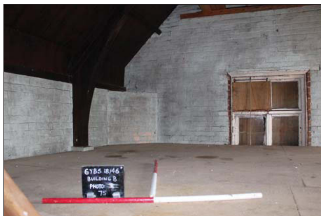
Plate 36. Former School, loft, View to angled corner showing roof truss, looking S, Scales: 2x 1m.
