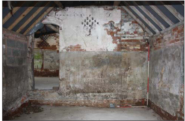
Plate 26. Barn C, interior, detail of party wall with Barn B, looking north-west. Scales: 2m, 1m.
