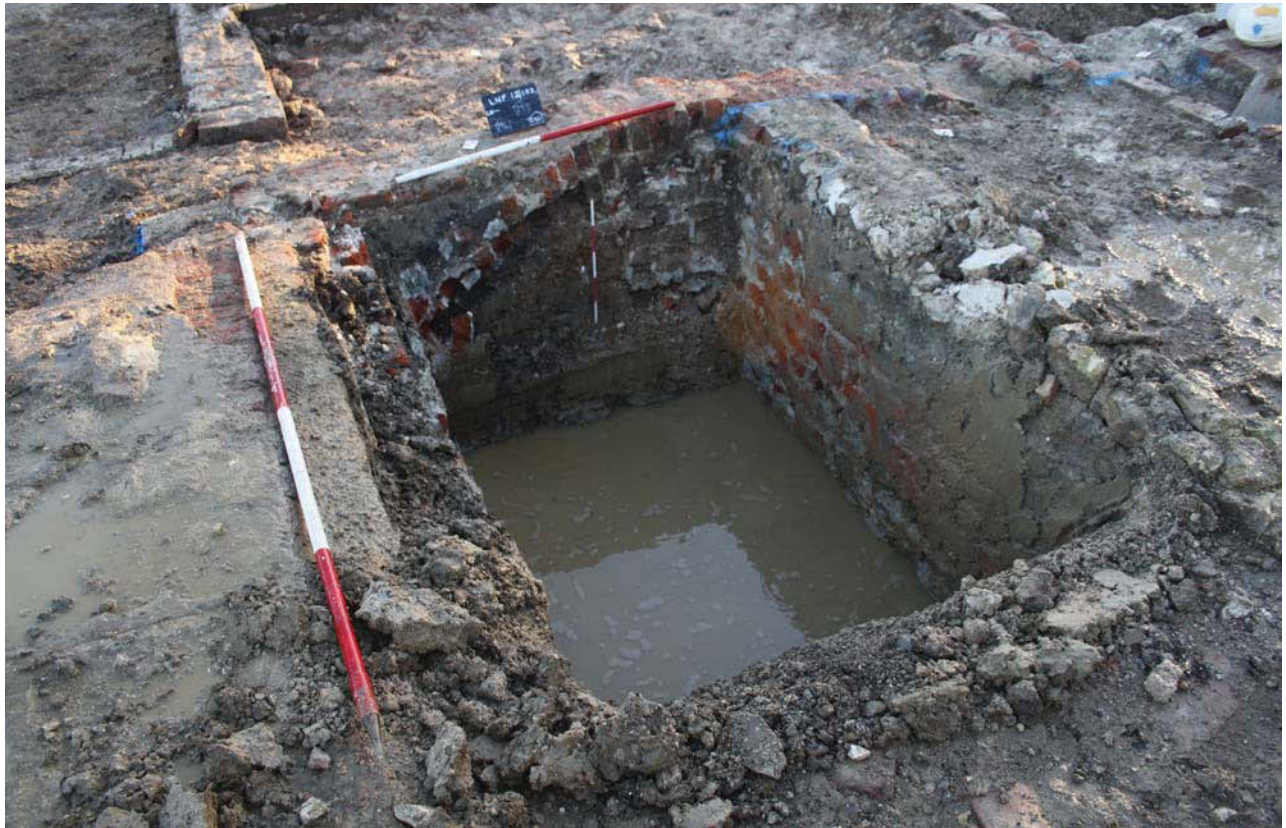
Plate 6. Cellar arch 291 and associated walls, looking west. Scales: horizontal 2m, 1m; vertical 0.5m.
