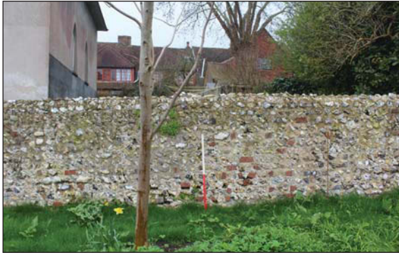
Plate 7. East side of wall showing later 'bungaroosh' construction, looking West. Scale: 1m.
