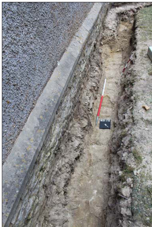
Plate 2. Underlying stone foundation (wall 150) to East Chancel wall, looking north, Scales: horizontal 1m, vertical 0.5m.
