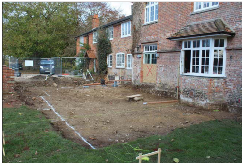
Plate 1. Extent of reduced for new extension, prior to footings, looking north east.
