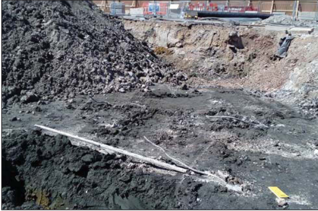
Plate 1. The surface of the alluvial clay exposed during remediation work in the centre of the site, looking north-west.
