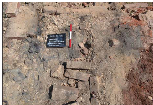
Plate 15. Boundary wall after demolition, remains of stone wall, looking east, Scale: 0.3m.
