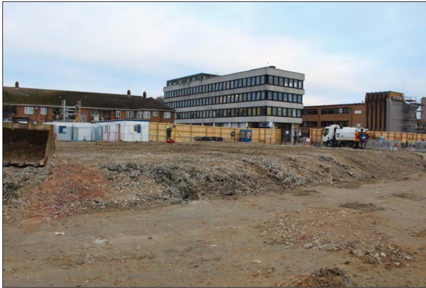
Plate 1. Area C and D, Levelling and inclusion of piling mat, looking north east.
