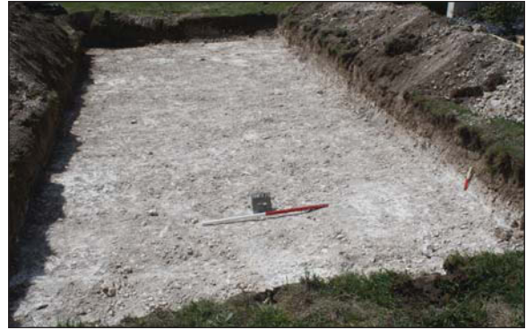
Plate 2. Area stripped for new swimming pool, looking West. Scales: 1m and 0.20m.
