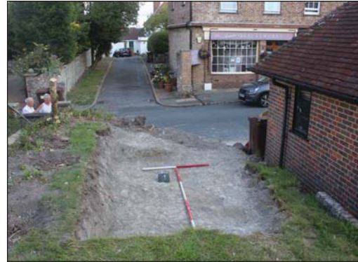
Plate 2. Area stripped in front garden, looking North. Scales: 2m, 1m and 0.30m.
