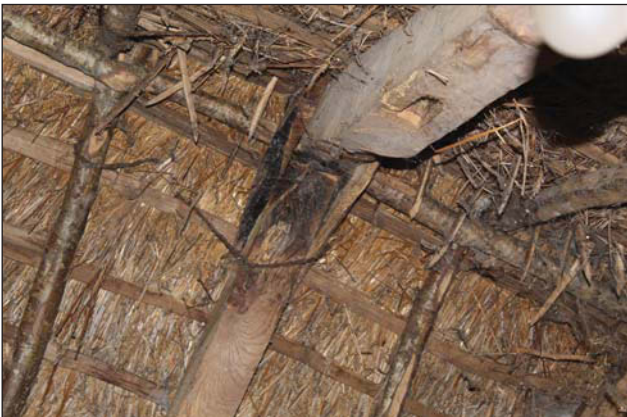
Plate 19. Blackened apex on truss in roof space.
