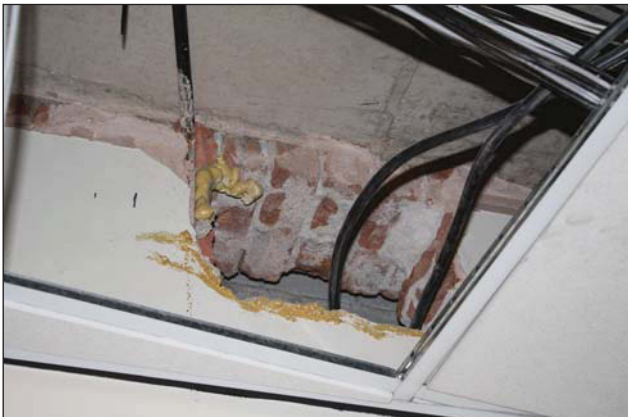
Plate 19. Ground floor, hole in wall, looking NW.
