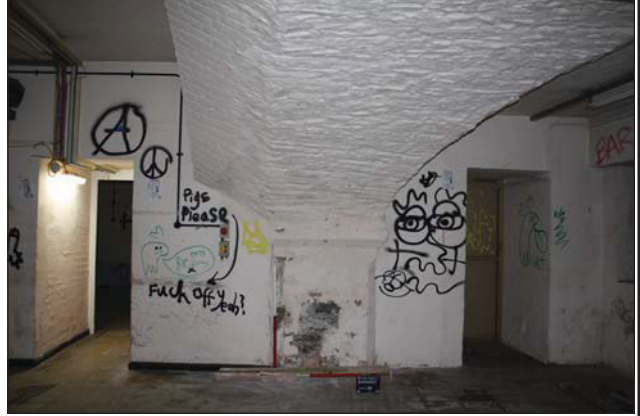
Plate 58. Lower ground 1, pier detail and brickwork in arch, looking NW, Scales: 2 x 1m.
