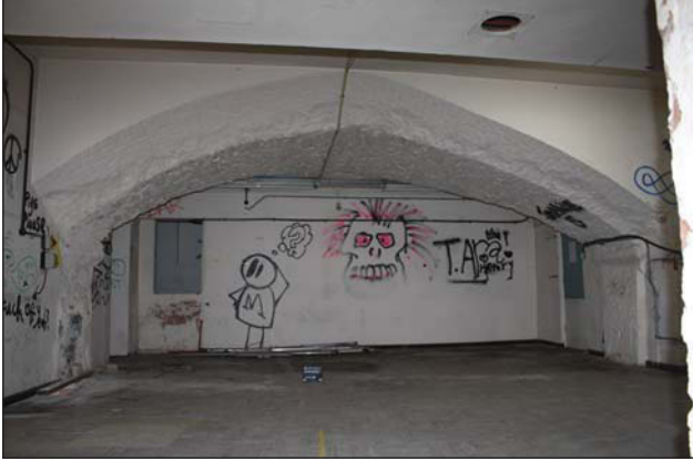
Plate 57. View to rear of undercroft, (lower ground 1), looking NE, Scales: 2 x 1m.
