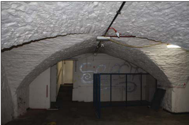
Plate 11. View to rear of undercroft, lower ground 1, looking NE, Scales: 2 x 1m.
