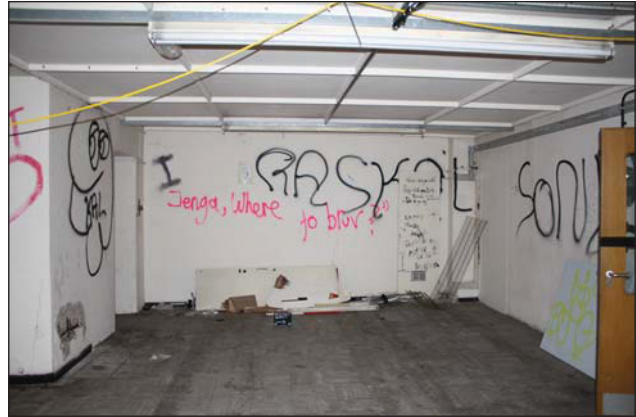
Plate 34. View to rear of cellar, lower ground 1, looking NE, Scales: 2 x 1m.
