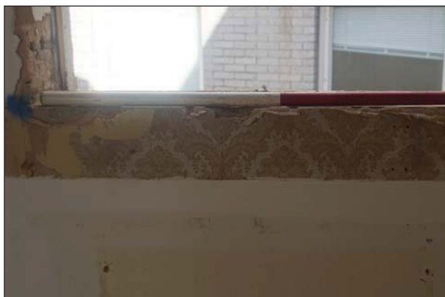
Plate 100. Wall paper detail, looking NE, Scales 1 x 1m.
