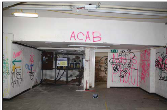
Plate 56. Lower ground 1, view to modernized front of undercroft, looking SW, Scales: 2 x 1m.
