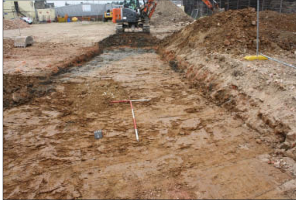
Plate 1. Reduction for the attenuation tank, central area, looking S, Scales: 2m and 1m.
