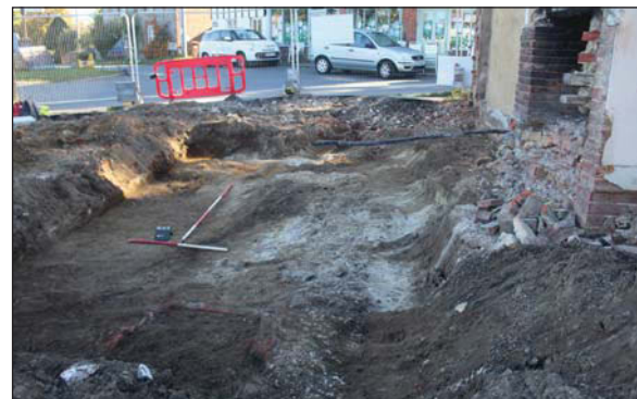
Plate 4. General view of eastern excavation area, looking East, showing features 1001, 250 and 102. Scales: 2m and 1m.
