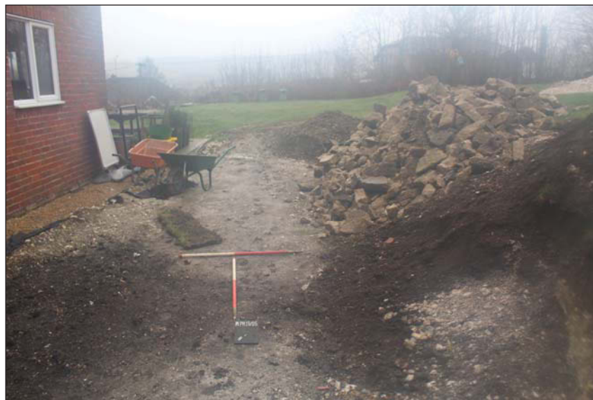
Plate 2. Ground reduction for access to rear of existing house, looking south east, Scales: 1m x2.
