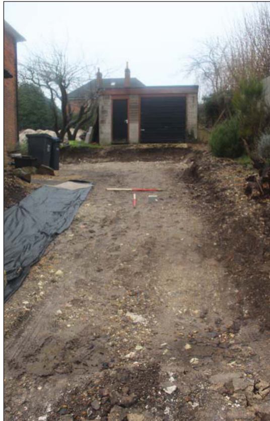
Plate 1. Ground reduction under previous concrete drive, looking south west, Scales: 1m x2.
