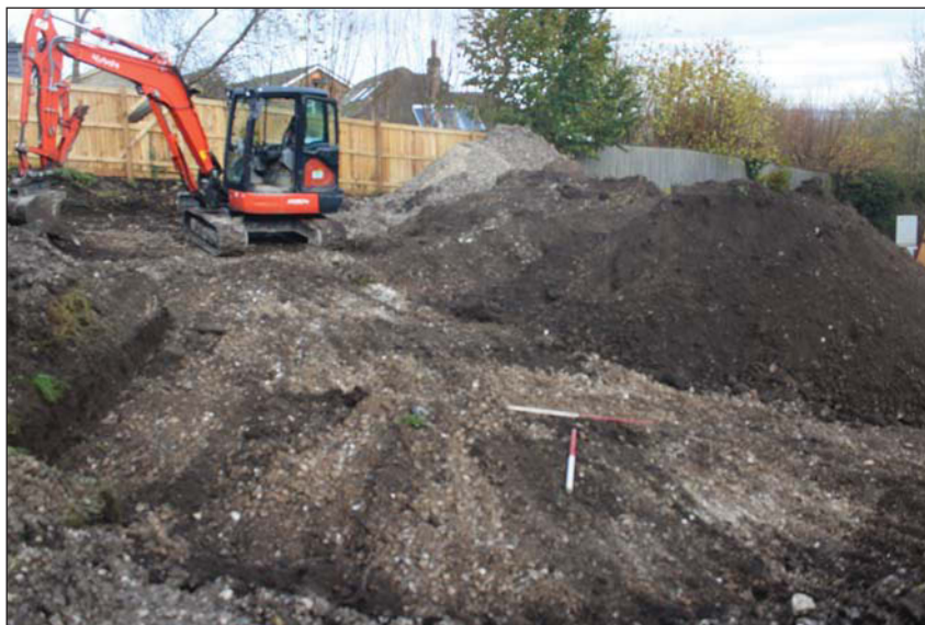
Plate 4. Ground reduction in garden area to west, looking south west, Scales: 1m x2.
