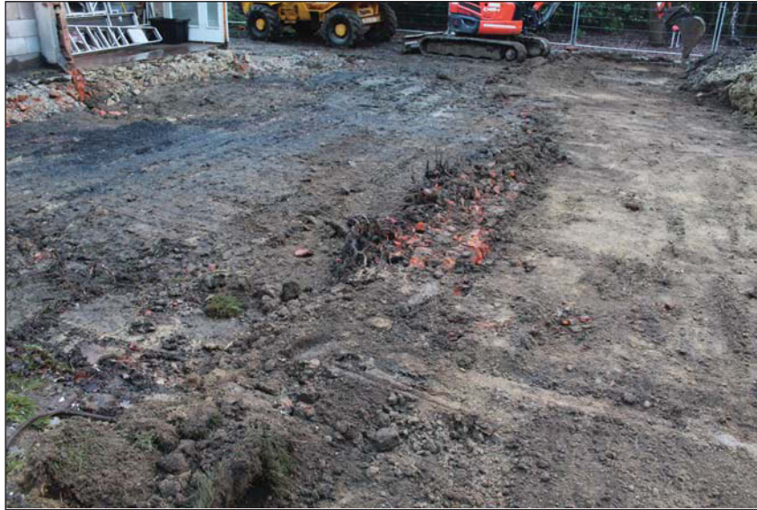
Plate 3. Stripped area following partial demolition of south of existing building looking East
