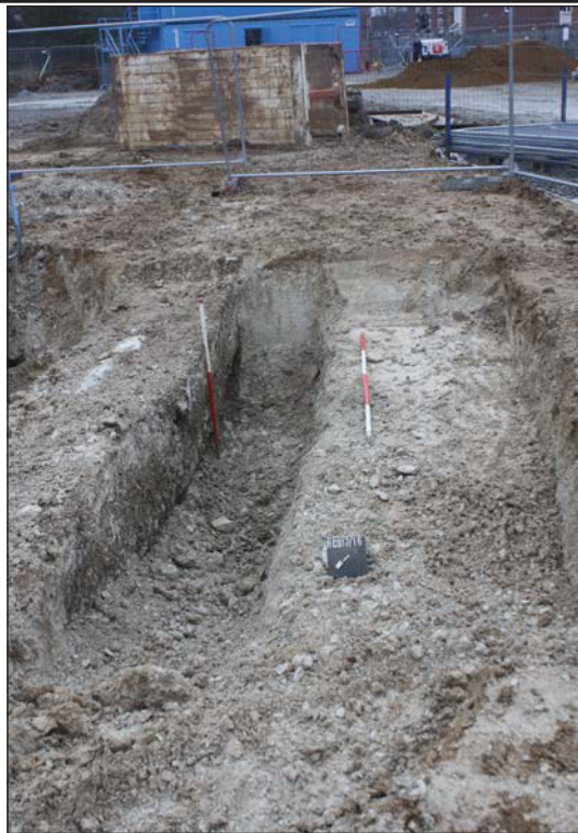
Plate 3. Stepped trench located on route of pipe trench, looking South East, Scales: 2m and 1m.
