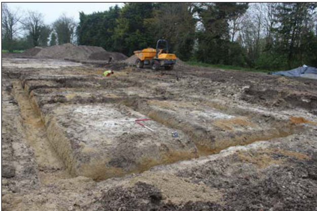
Plate 7. Working shot of Barn D foundation trenches, looking North West, Scales: 2x1m
