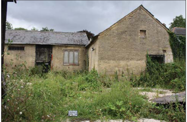
Plate 46. North elevation and gable end of building A, looking S, Scales: 1x1m, 1x2m.
