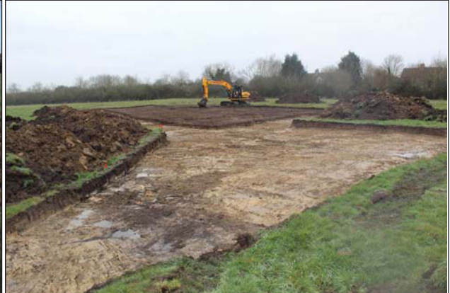
Plate 2. Ditch partially backfilled during modern era, still visible in landscape, looking South West.
