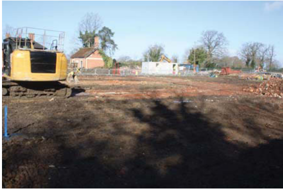
Plate 1. Area strip for First Team Building. Site of former greenhouses, looking west
