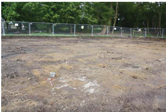
Plate 5. Area strip of First Team Building NE corner, looking NE, Scales 0.50m and 0.30m
