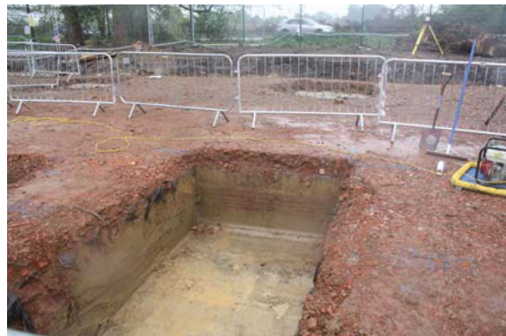
Plate 4. Footing at the west end of the footprint of the First Team Building, looking west
