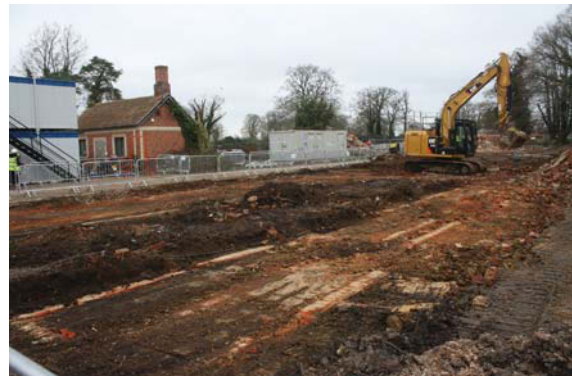
Plate 6. Area strip of First Team Building showing former greenhouse foundations, looking SE
