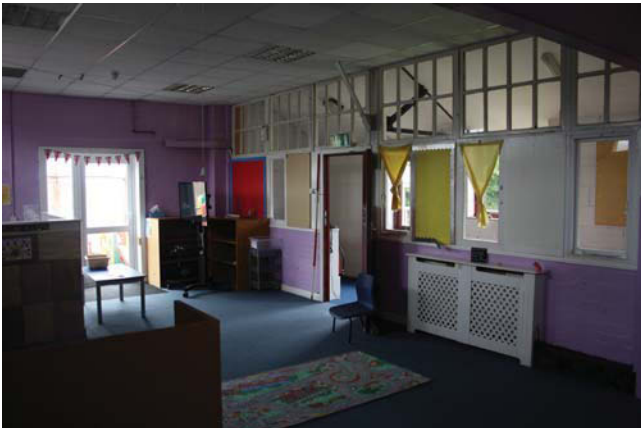
Plate 29. Nursery Room 6: general view to internal windows, looking south-east, Scales: 2m and 1m.
