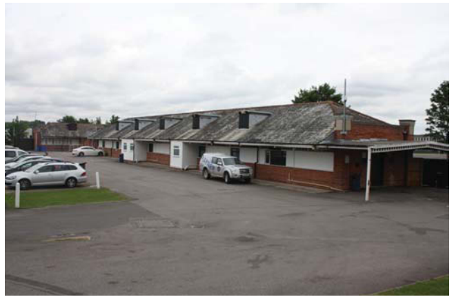
Plate 24. Nursery: oblique view of West elevation, looking north-east, Scales: 2m and 1m.
