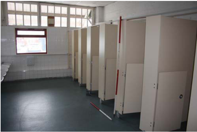
Plate 33. Nursery Room 10: toilet view old wall, looking north-west, Scales: 2m and 1m.
