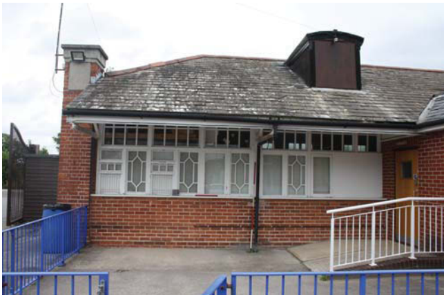
Plate 19. Nursery: south elevation (E – W building), looking east, Scales: 2m and 1m.
