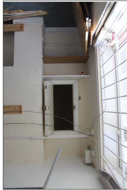
Plate 26. Office G-005 towards hatch opening to the public access lobby, looking S
