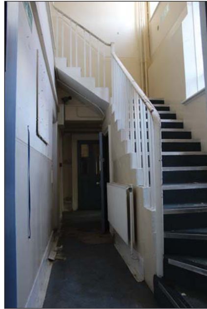
Plate 22. Stair well to 1st floor from door of corridor G-031, looking E.
