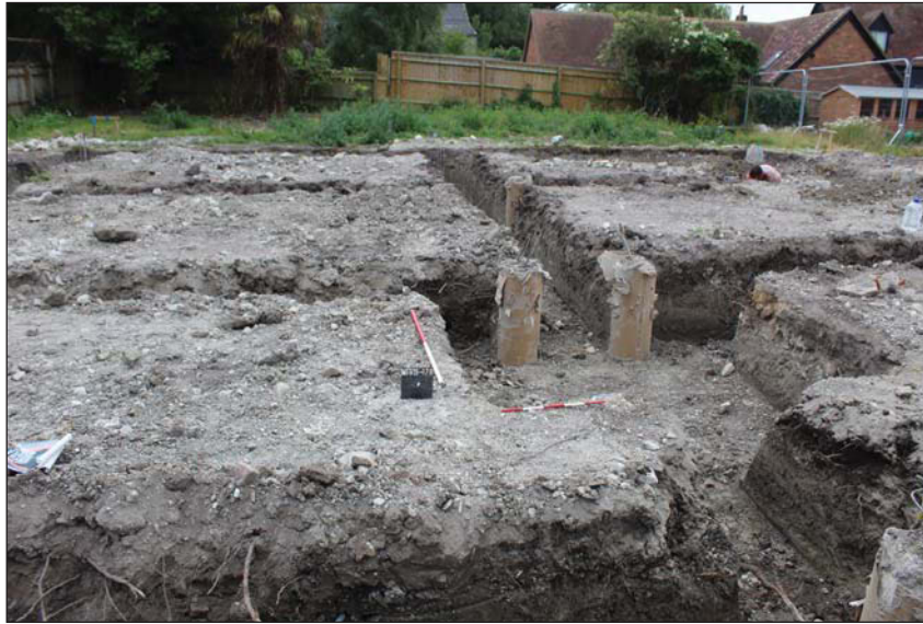
Plate 1. View through central excavation of new footings, looking south, Scales: 1m and 0.5m.
