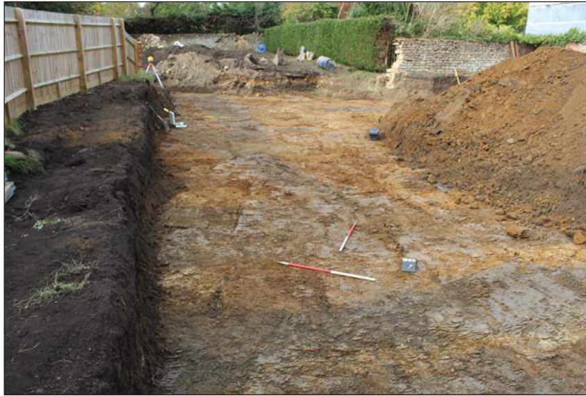
Plate 3. Formation level stripped in south east, looking North West, Scales: 1m x2.
