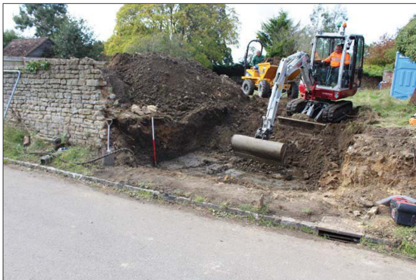
Plate 2. Excavation of new access and ground reduction, looking South West, Scale: 1m.
