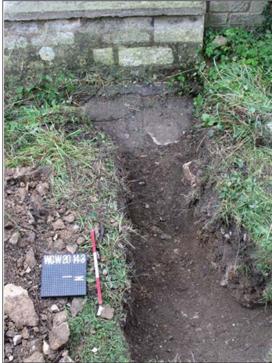
Plate 1. Connection of new drainage trench to north aisle wall, looking S, Scale: 0.3m.
