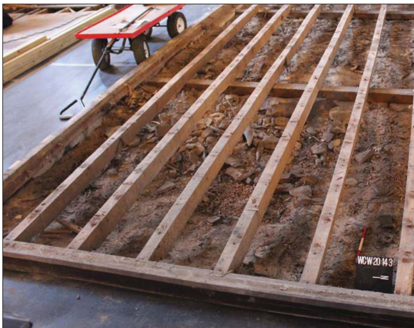
Plate 4. Exposure of void on north side of the western nave suspended floor, Scale: 0.3m.
