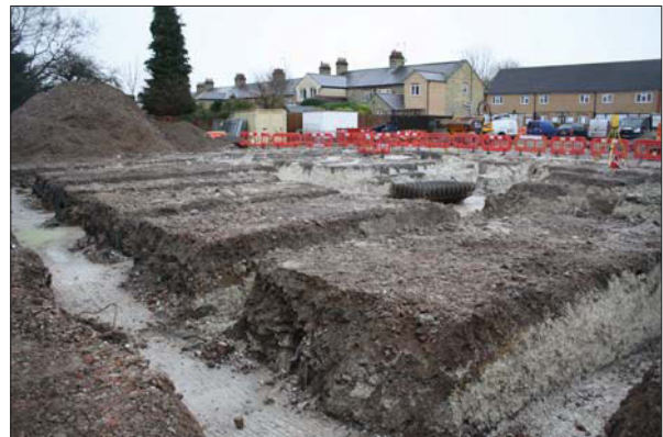
Plate 8. View of new footings, showing the varying depth of made ground overlaying geology.
