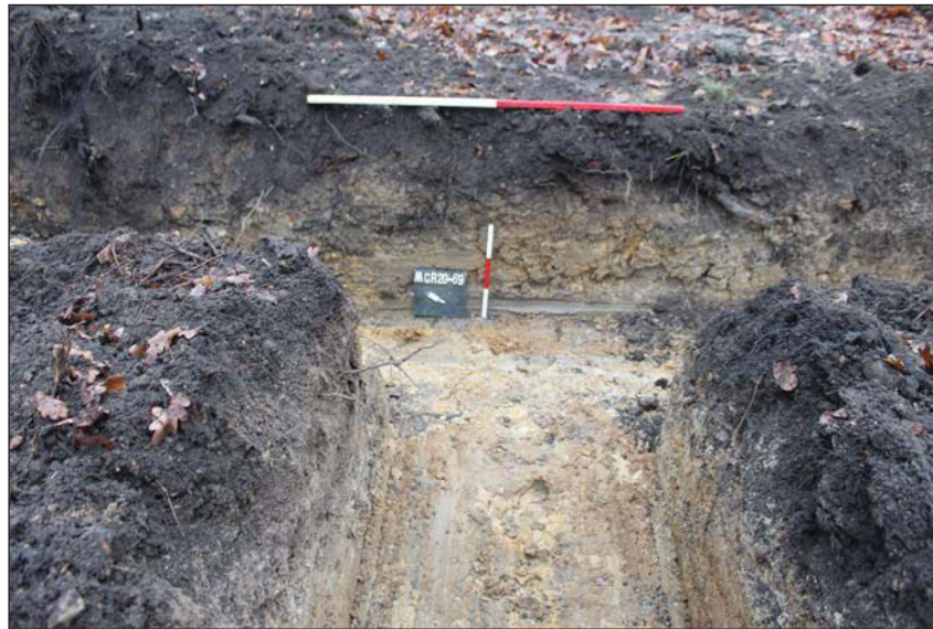
Plate 3. View at base of excavated footings, looking North East, Scales: 1m and 0.3m.
