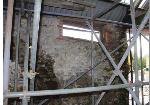
Plate 70. Close up of window next to south eastern doorway, wooden lintel and red brick frame. Looking South East.
