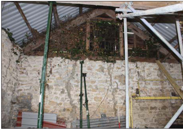
Plate 61. North eastern wall of main barn. Stone wall with wooden gable frame, with hay loft hatch. Looking North East. Scale: 1m
