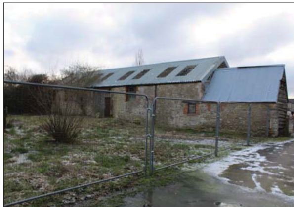
Plate 21. General view of north western elevation and lean-to, steel roof, windows and north western doorway visible. Looking East. Scale: 1m
