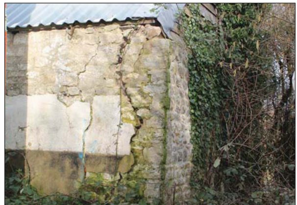
Plate 54. Close up of eastern corner of barn with cracks and render on the stone wall. Looking West.
