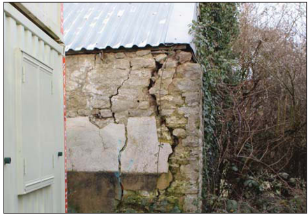
Plate 4. South eastern outer corner of barn, large cracks in the corner. Looking North West
