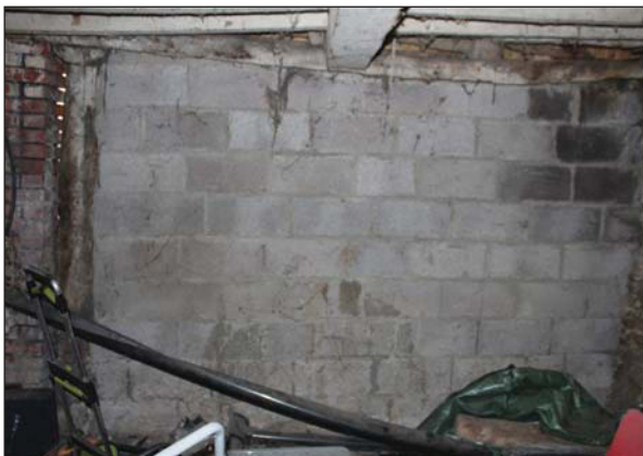
Plate 53. Interior breeze block wall in south western barn chamber. Looking South West.
