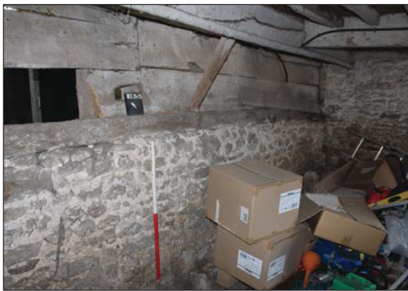
Plate 51. Interior wall of south western chamber of barn. Stone wall with wooden slats. Looking East. Scale: 1m
