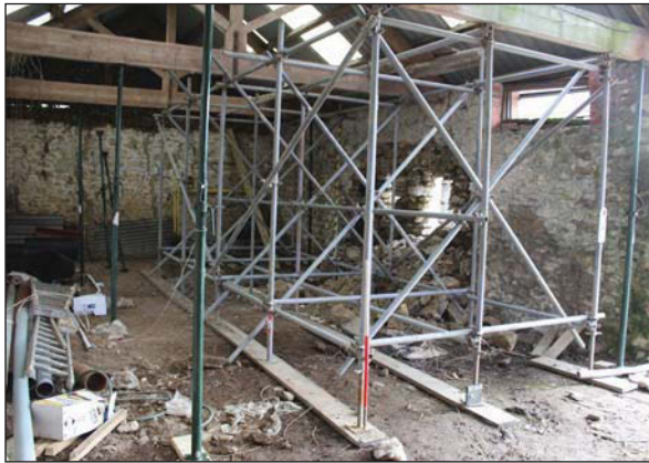
Plat 57. Damaged south western interior wall, rubble and gaps. Looking East. Scale: 1m
