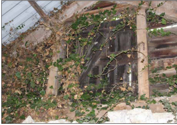
Plate 73, Ivy over growing hay loft hatch. Looking North.
