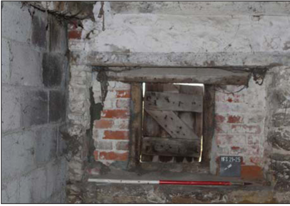
Plate 49. Close up of north west wall of chamber, interior view of south western most window, with wooden lintel and shutter. Looking North West. Scale: 1m
