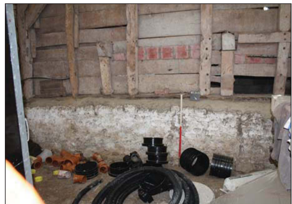
Plate 76. South west end of barn. Interior stone and wood wall, with wooden supports. Looking South West. Scale: 1m
