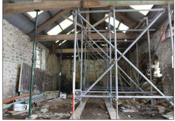
Plate 56. Interior of main barn. Damage to south eastern wall shown. Scaffolding holding up roof. Large glass window in north western wall. A frame wooden supports for steel roof. Looking North East. Scale: 1m
