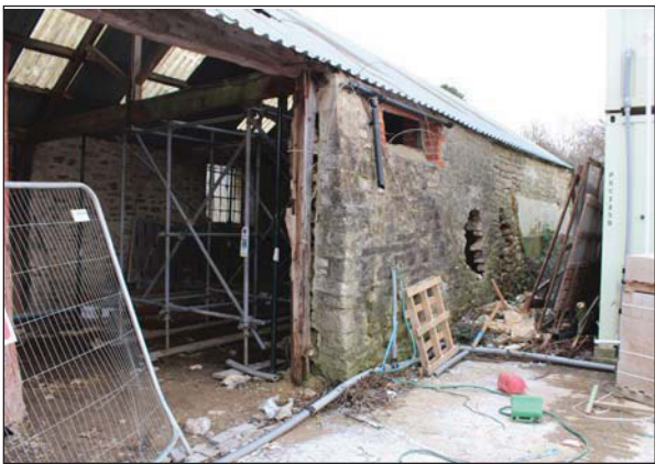
Plate 3. Barn door with nearby window and damage to the wall. Looking North
