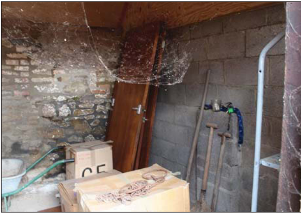
Plate 43. North corner of lean-to. Breeze block dividing wall and interior of north west wall. Looking North.
