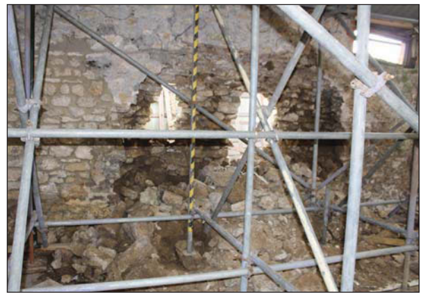
Plate 64. Close up of interior damage to south eastern wall, two large holes with stone rubble. Looking South East.
