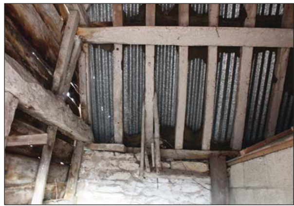
Plate 34. Interior roof of lean-to. Wooden beams and rafters supporting the corrugated steel roof. Looking North West.
