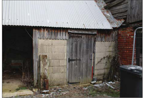
Plate 14. View of south east elevation on lean-to wall, both wooden doors and steel roof. Looking North West. Scale: 1m
