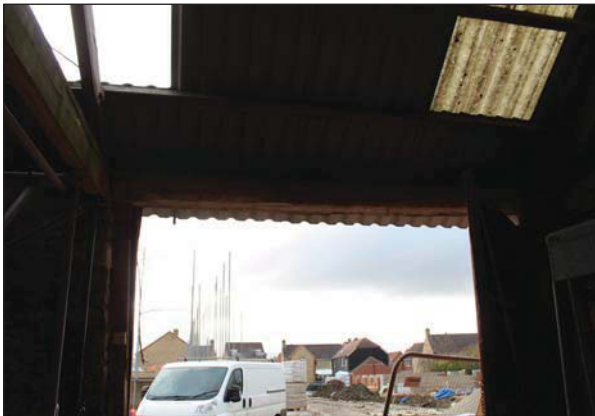
Plate 83. View out of south eastern doorway showing wooden lintel and stone frame. Looking South East.
