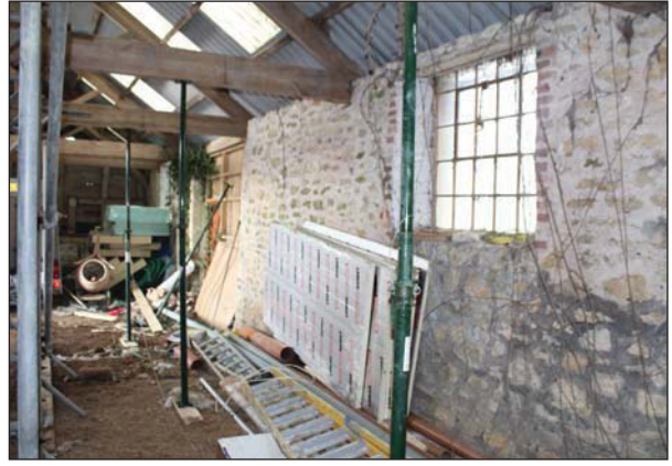
Plate 68. View of interior north western wall, glass window and doorway present. Looking West.
