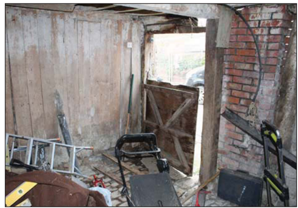
Plate 46. Inside of south western chamber looking out, half wooden door visible. Looking South.
