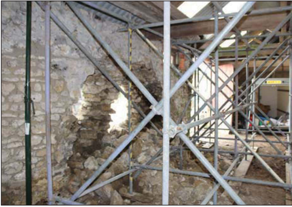
Plate 67. View of damage on south eastern wall. Looking South.
