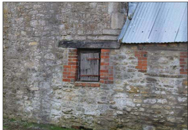
Plate 22. Close up of north western hatch window, wooden lintel and shutter. Looking East.
