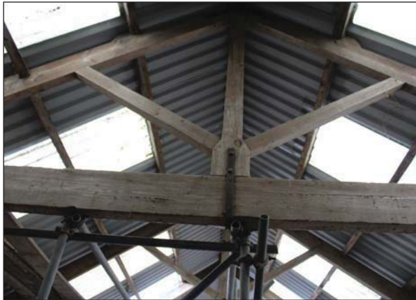
Plate 69. Close up of roofs wooden frame supporting the steel roof and skylights. Looking South West.
