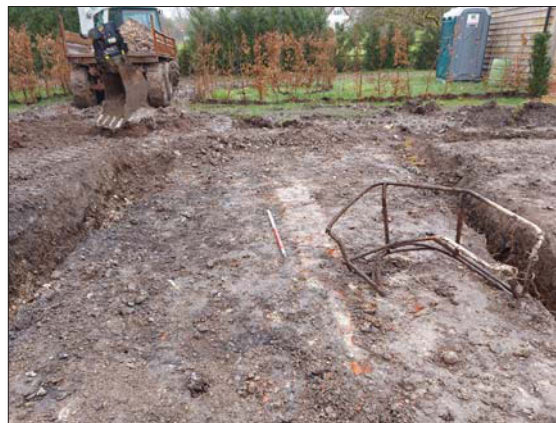
Plate 2. Single course brick at base of overburden strip, looking East, Scale: 1m.
