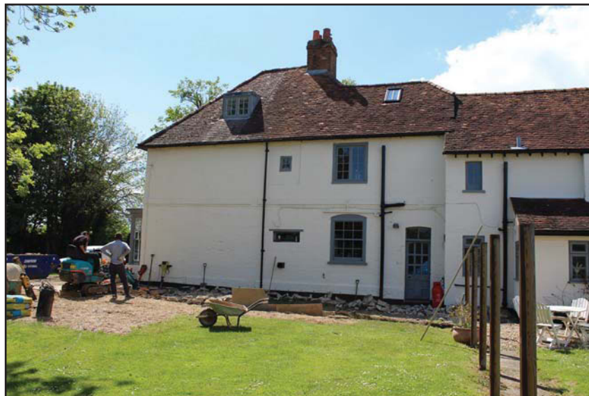
Plate 1. Footing trenches under excavation on the east side of the building, looking west.
