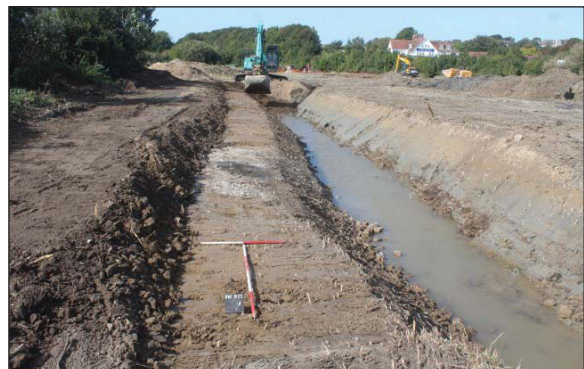
Plate 6. Excavation of new watercourse at Shoreham Airfield, looking North-west. Scales: 2m and 1m.
