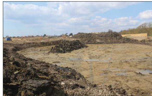
Plate 4. General view of area stripped for a new reed bed, looking West.
