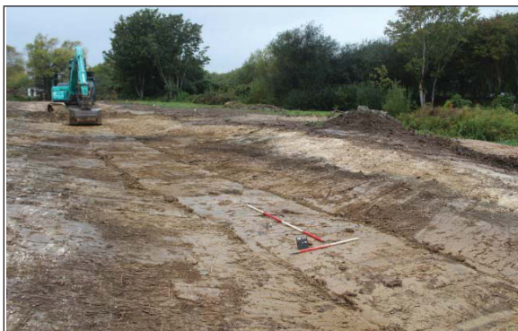
Plate 5. Excavation of new watercourse at Shoreham Airfield, looking North-west. Scales: 2m and 1m.
