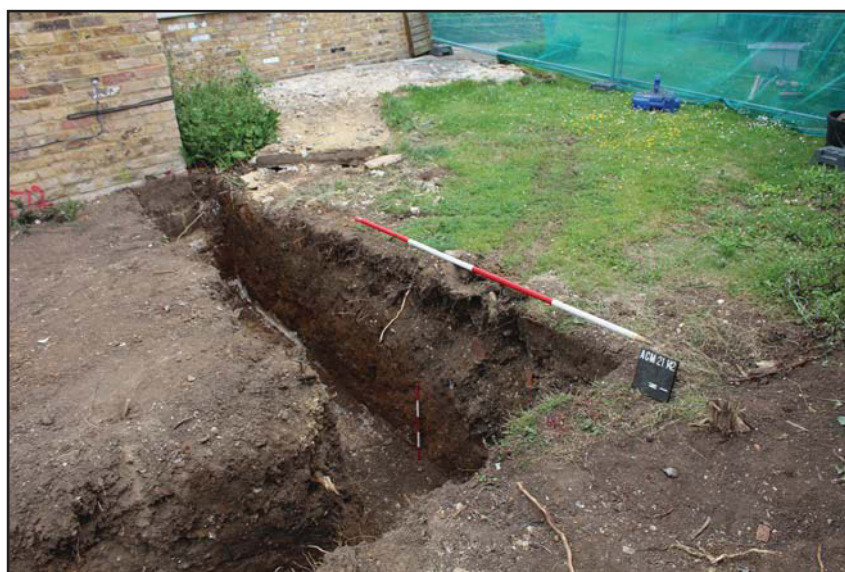
Plate 2. Foundation trench at eastern area of extension, looking north east, Scales: 2m and 0.5m.
