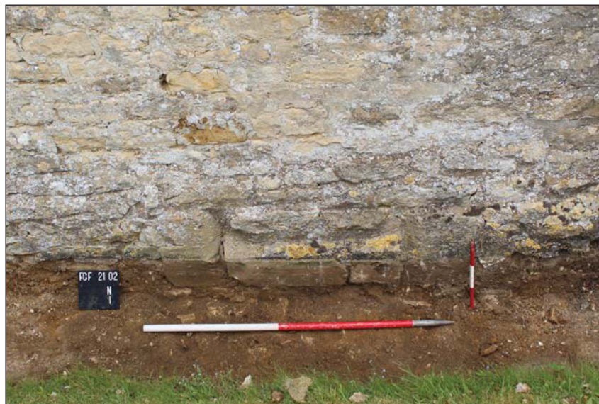
Plate 2. South circuit drain, Detail of former doorway, looking North, Scales: horizontal 1m, vertical 0.3m.
