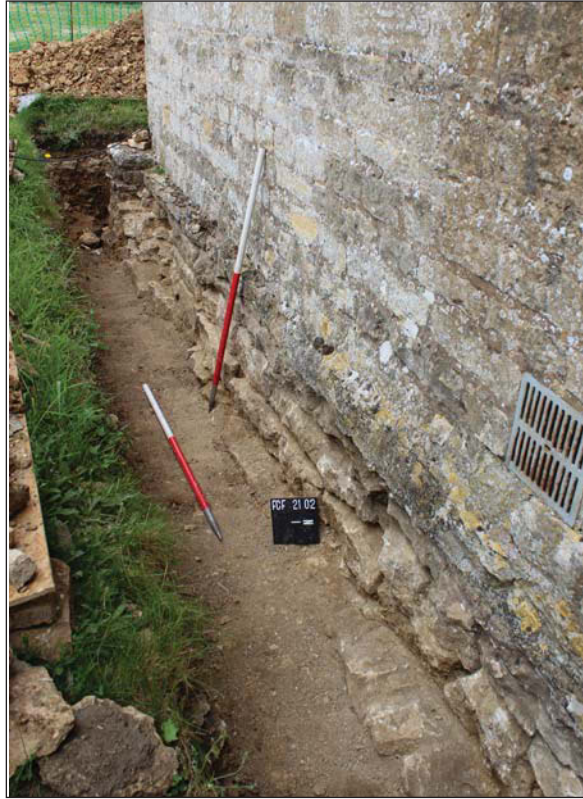
Plate 5. South circuit drain, South west corner nave foundation, looking West, Scales: horizontal 1m, vertical 1m.
