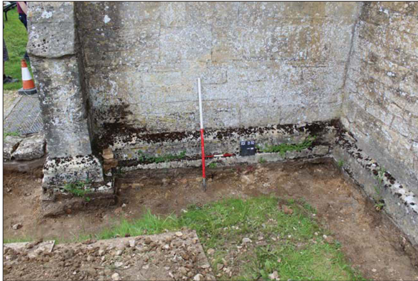
Plate 3. South circuit trench, Exposed foundation, south porch, looking west, Scales: horizontal 0.3m, vertical 1m.
