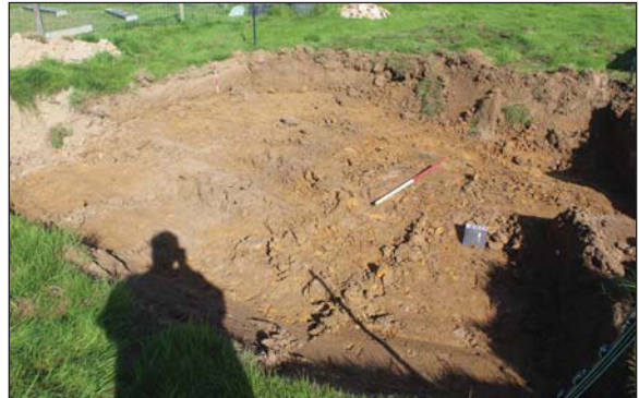
Plate 6. General view of area stripped for attenuation tank, looking North-west. Scales: 1m and 0.50m.
