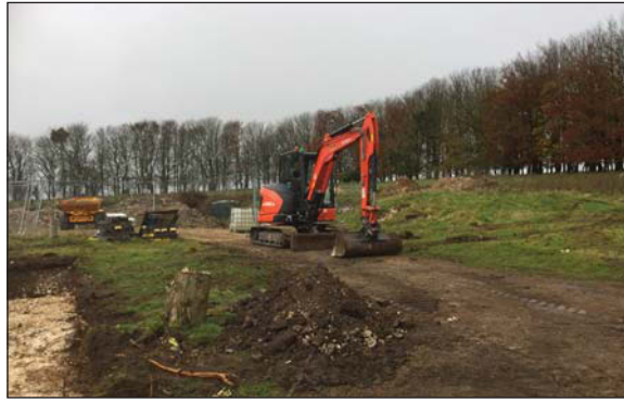
Plate 9. General view of site, looking West from the eastern end of trench 1.
