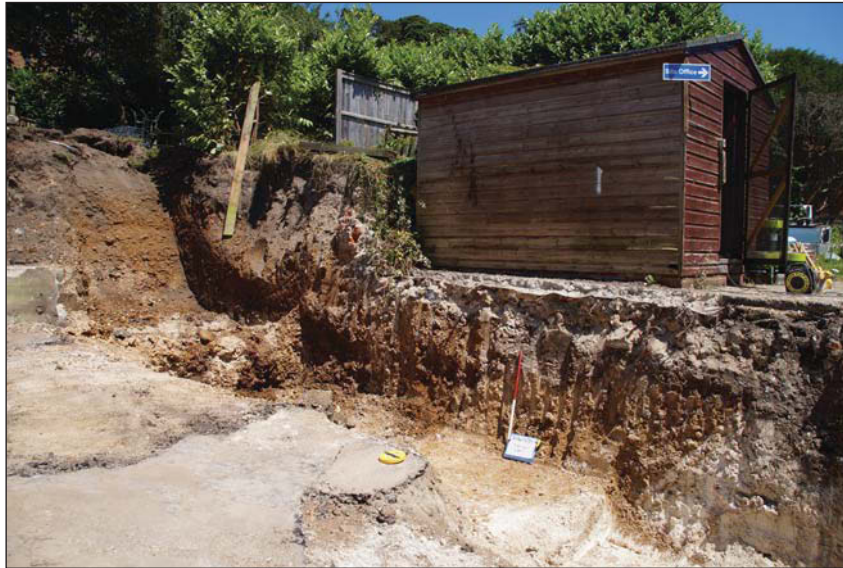
Plate 3. Exposed section excavating the new stairs to north of site, looking north east, Scale: 1m.
