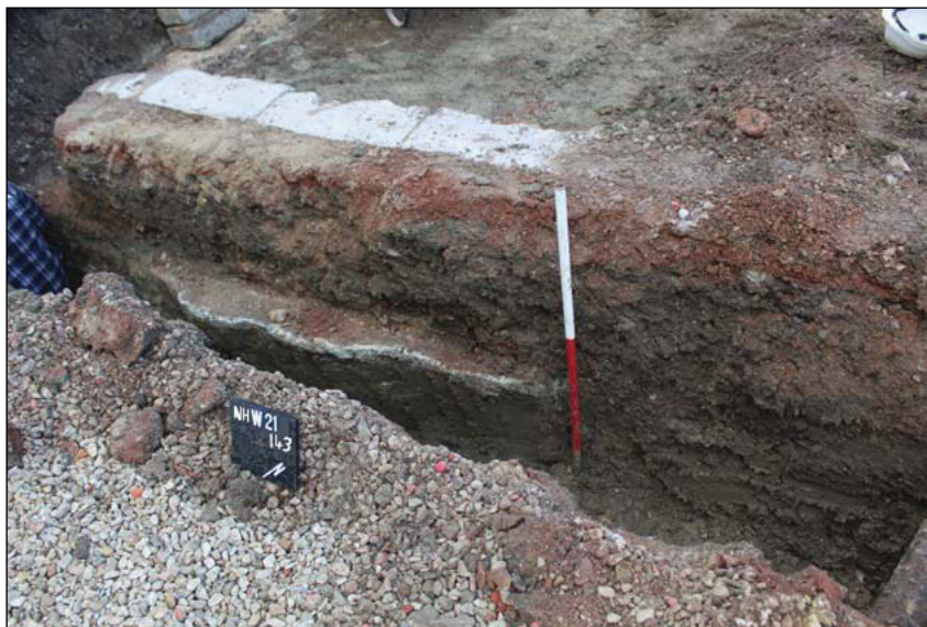
Plate 4. Truncation of previous foundation in East side trench section, looking South West, Scale: 1m.
