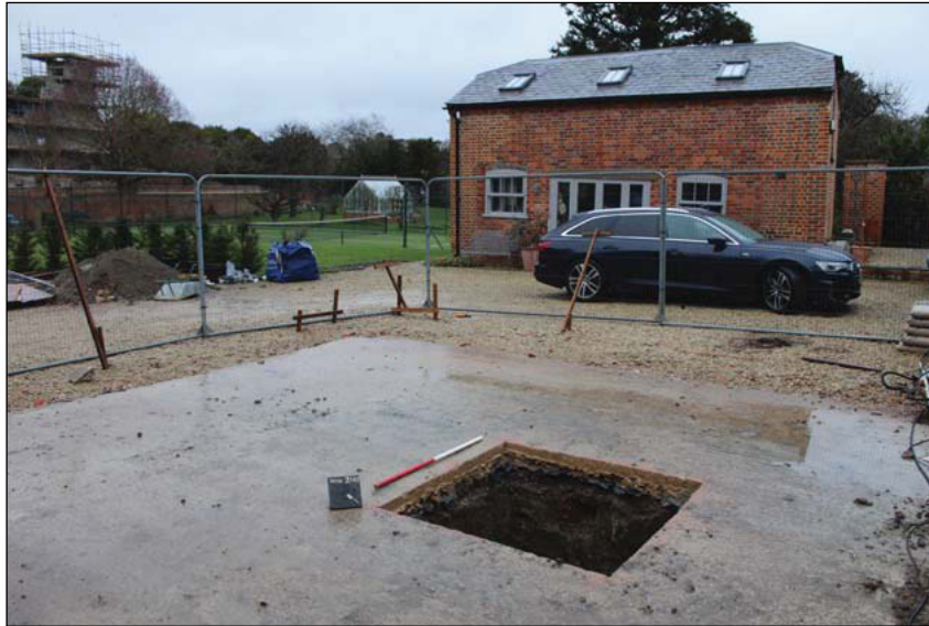
Plate 1. Setting, showing Test Pit before concrete slab removed, looking North East, Scale: 1m.
