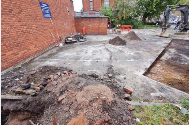
Plate 1. View of site showing trench to right, corner of test pit 1 bottom left and test pit 2 top left, looking north.
