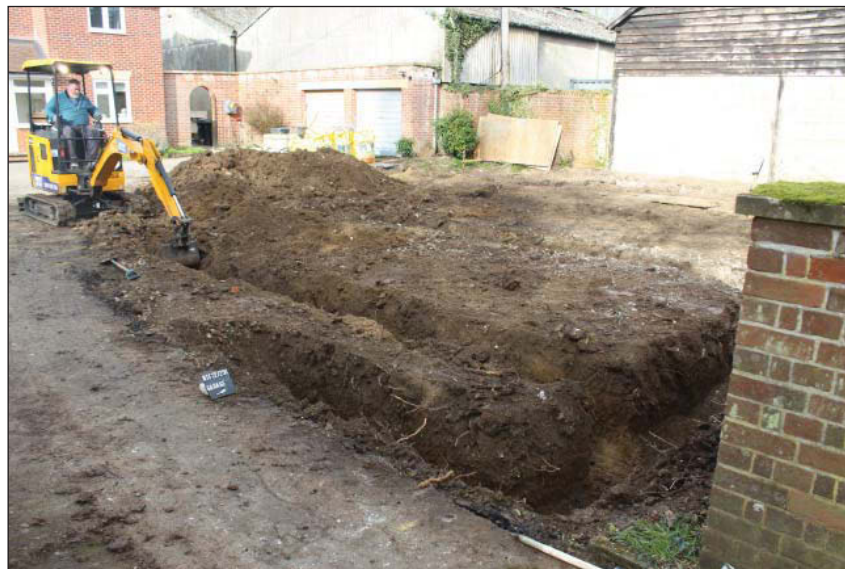
Plate 1. View of site, looking northwest across the footings of the new garage.
