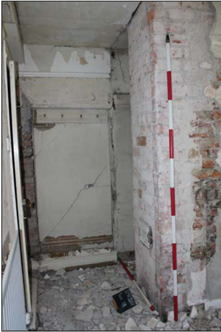
Plate 5. Looking north at the blocked up opening to the side of the chimney on the first floor, Scales: 2m and 1m.
