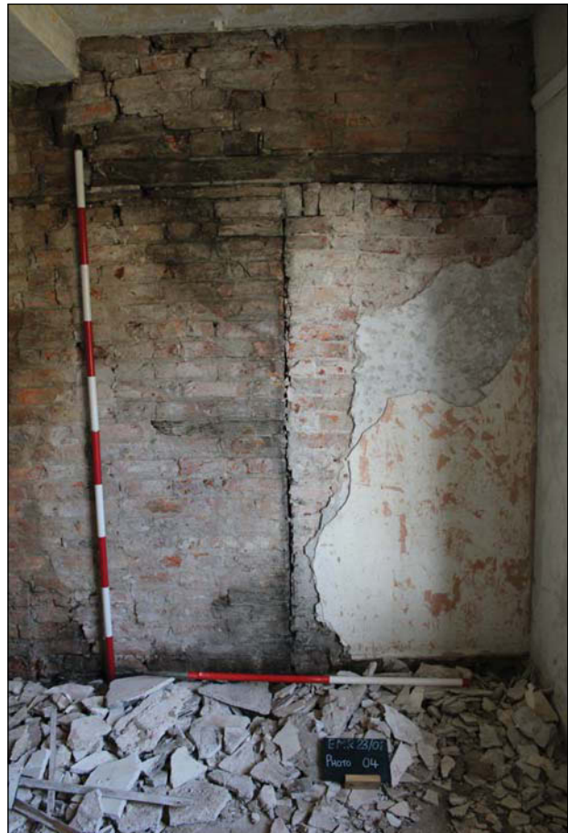
Plate 4. Looking north at the blocked up door on the first floor, Scales: 2m and 1m.
