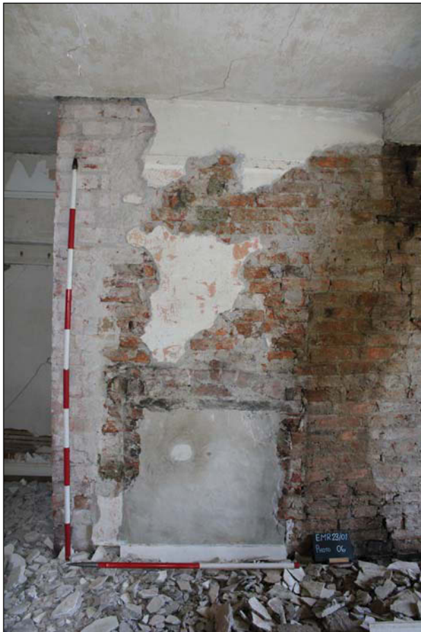
Plate 3. Looking north at the blocked up fireplace on the first floor, Scales: 2m and 1m.
