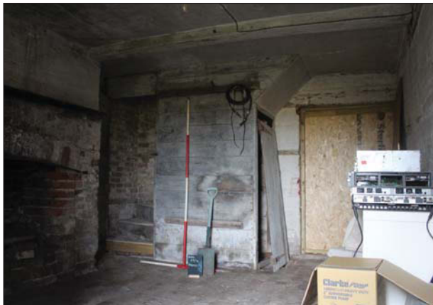
Plate 11. Main building 1: View to stairs and external door looking South East, Scales: 1x1m, 1x2m.
