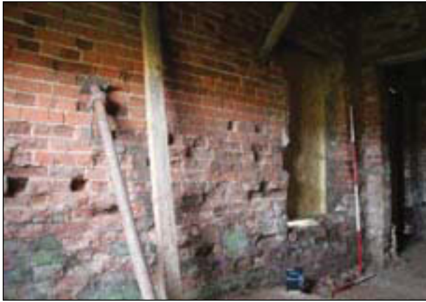
Plate 61. Rear building: Oblique of east wall, looking south-east Scales: 2m and 1m.
