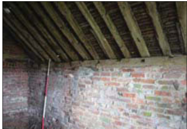
Plate 60. Rear building: Along wall plate on west wall, looking south-west, Scales: 2m.
