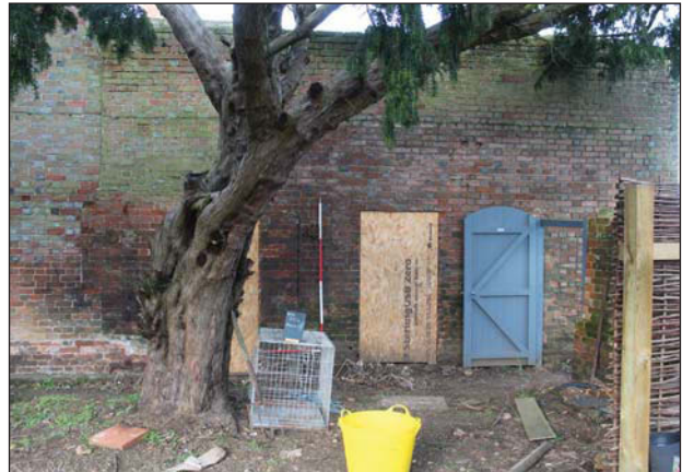
Plate 10. External: Rear building and rear link, east elevation looking West, Scales: 1x1m, 1x2m
