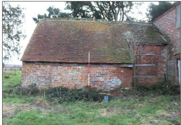
Plate 56. External: Rear building and rear link, west elevation, looking east, Scales: 2m and 1m.
