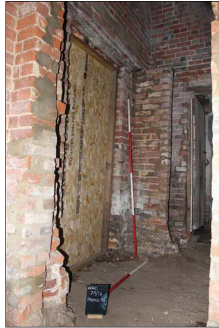
Plate 66. Rear link: Oblique east wall with doorway, looking south-east, Scales: 2m and 1m.
