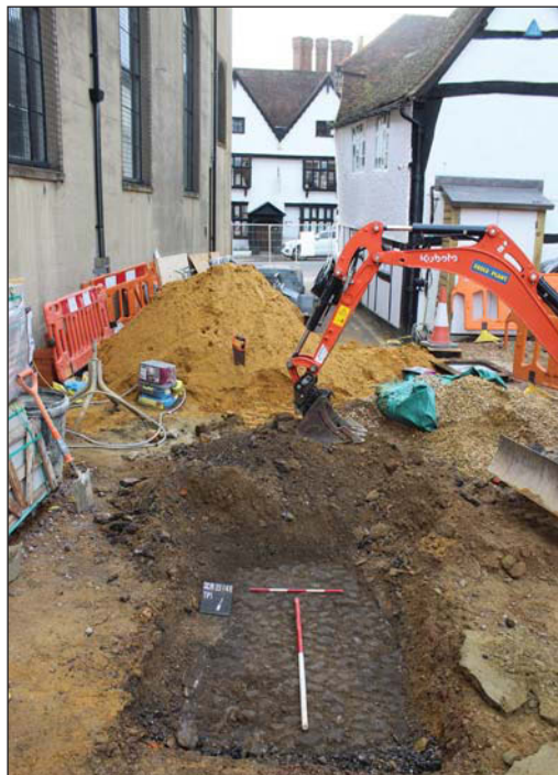
Plate 7. Preserved Cobbled Surface (50) within Test Pit 1, looking South-East, Scales: 1m and 0.5m.
