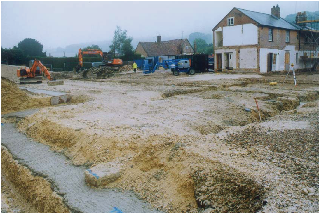
Plate 2. General view over new footings, with 19th century northern addition (rear) visible in the background.
