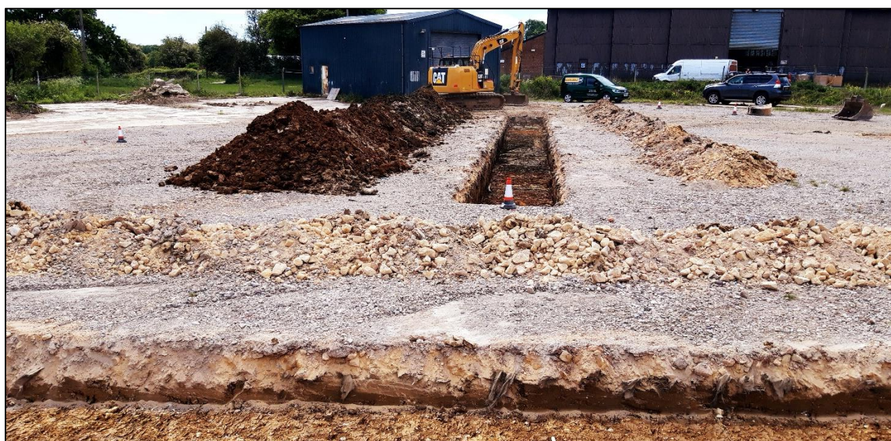
Plate 1 General shot of trenching in progress, looking SW across Trench 1 (foreground) and along Trench 3
