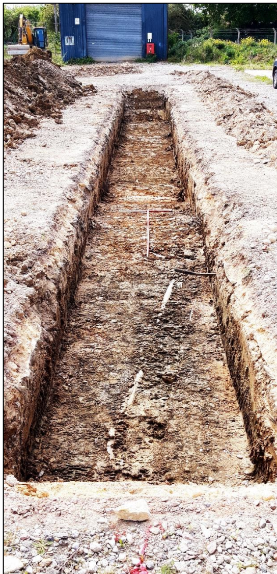
Plate 4 Trench 2 following machine excavation, revealing deep backfilled and levelling deposits criss-crossed by numerous service trenches.
