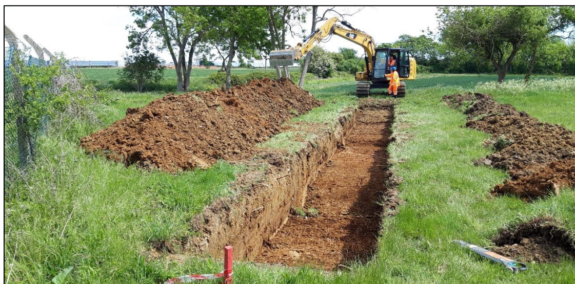
Plate 3 Trench 5 during machine excavation. This part of the Site lay within the former airfield curtilage, but outside of the area of concrete hardstanding.
