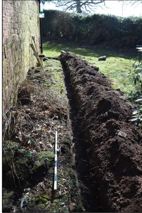
Fig. 4 View from the north of the trenching along the south-west elevation of the cafeteria. Photo CPAT 4482-0005
