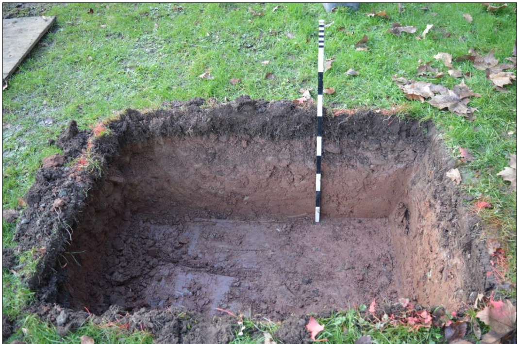
Fig. 5 Excavations for a junction box within the parkland, showing the shallow topsoil lying directly above the subsoil
