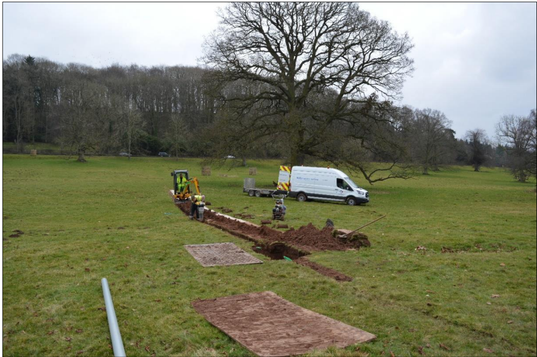
Fig. 4 Cable trenching at the point where the route crossed the ditch MNA 182188
